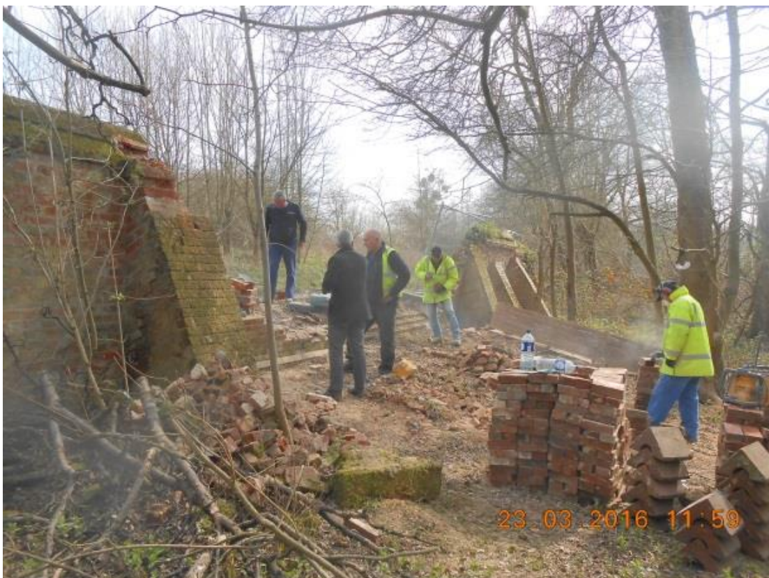
Fig. 6 – The repair of Braxted Park Wall is being funded by enabling development
